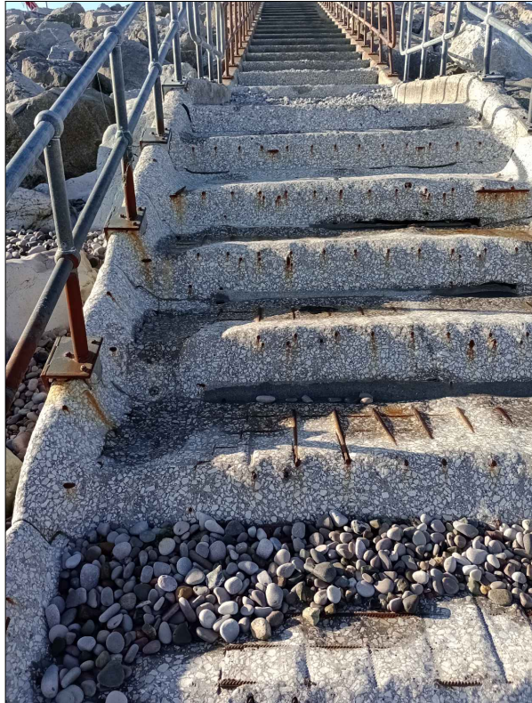
PHOTO 2 - VIEW OF EXPOSED REBAR ON LEFT OF STAIRCASE
