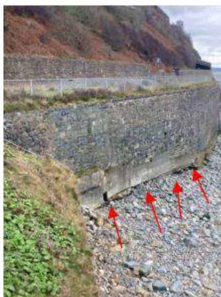
Figure 2 - Area of undermining, image taken from PPM Scoping Report - 1067_WAL_MPH - 01_03_2023.
