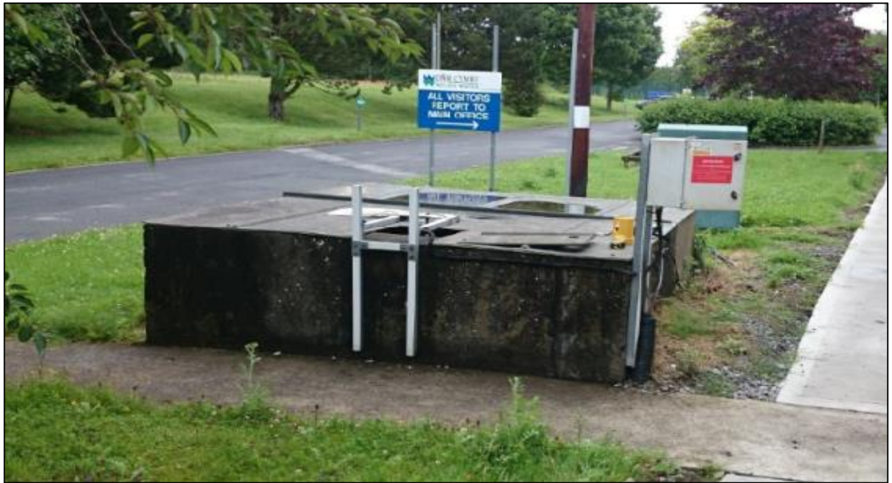
Figure 3: Image of the Storm Overflow Chamber
