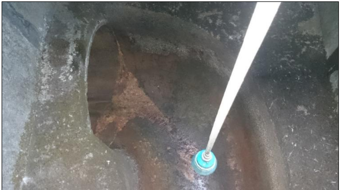
Figure 4: Image of the Level monitor in the Storm Overflow Chamber
