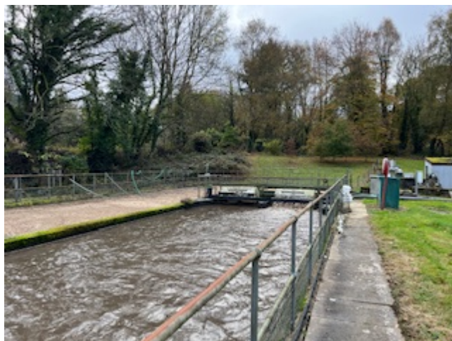
Image 2 – Aeration lane in operation.
