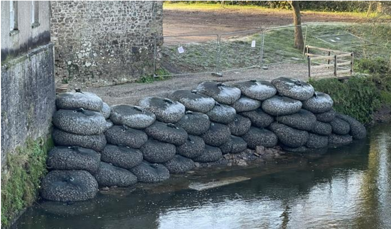
Figure 1-2: Emergency repair works to wall failure
