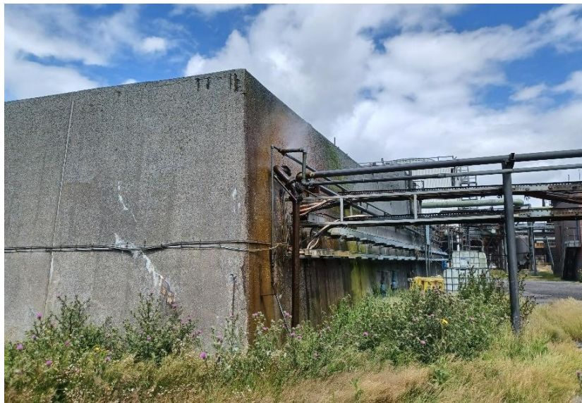
Image 4: Failed Water Inlet Pipe on BET Plant
