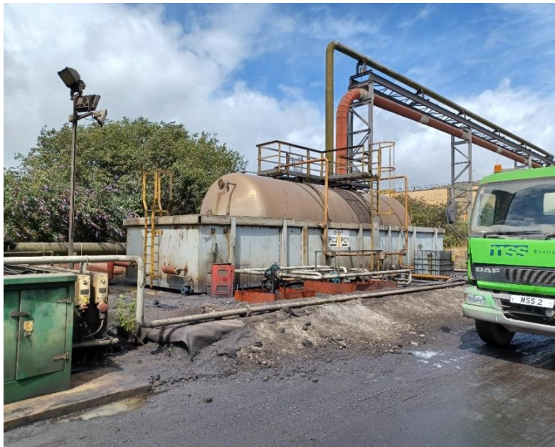
Image 6: Processed Oil Tank
