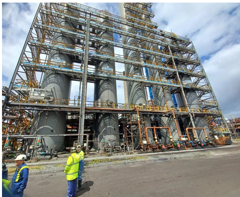
Image 2: Benzole, Ammonia and Naphthalene Washer Tanks
