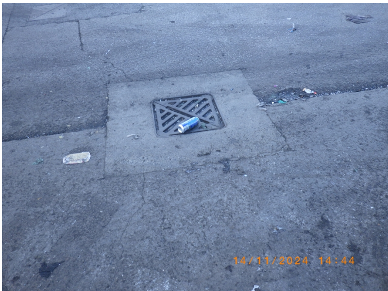
Image of drain at the rear of the site with debris in it.
