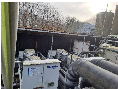
Image 4. Chillers x3, glycol pumps adjacent
