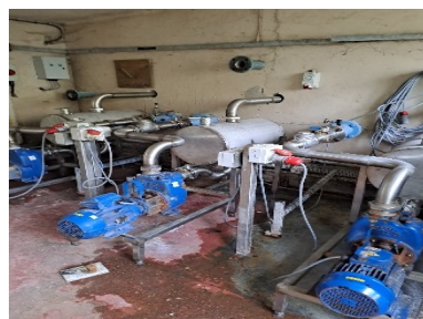
Image 4. Pump house (within a building)
