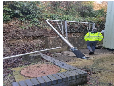
Image 13. Pipe system from ETP area to underground pipe out to emission point W1
