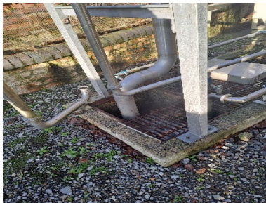
Image 12. ETP effluent to sump
