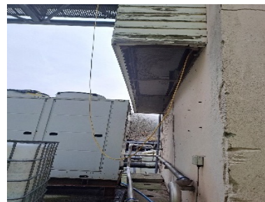
Image 3. Side of compressor room
