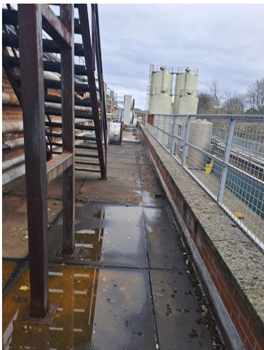
Cheese room outlet, vacuum pump room outlet and condenser fans (Image 8&9);
