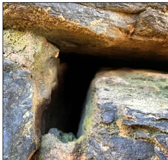
Figure 13: Cavity feature within northeast wingwall.
