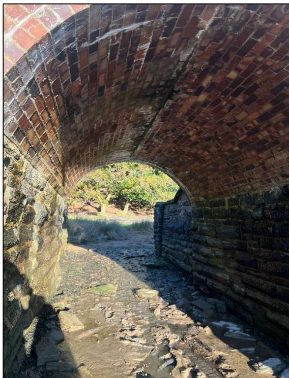
Figure 6: Masonry Arch of underbridge, with stress fracture observed.
