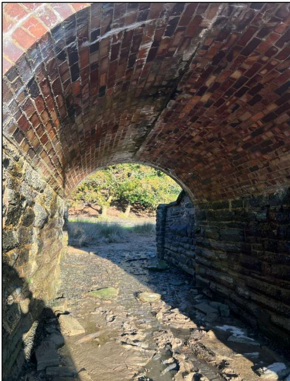
Figure 12: Masonry Arch of underbridge, with stress fracture observed.
