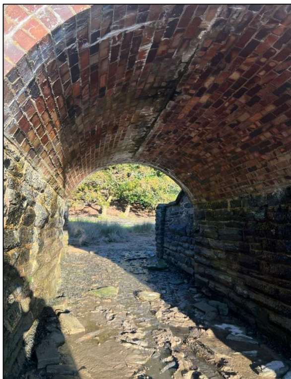
Figure 8: Masonry Arch of underbridge, with stress fracture observed.
