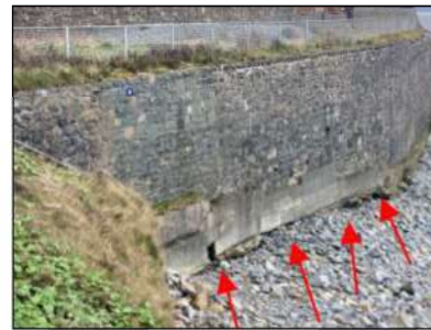
Photo 1—Area of wall undermining
