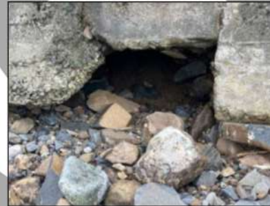
Photo 2— Close up of undermining extents
