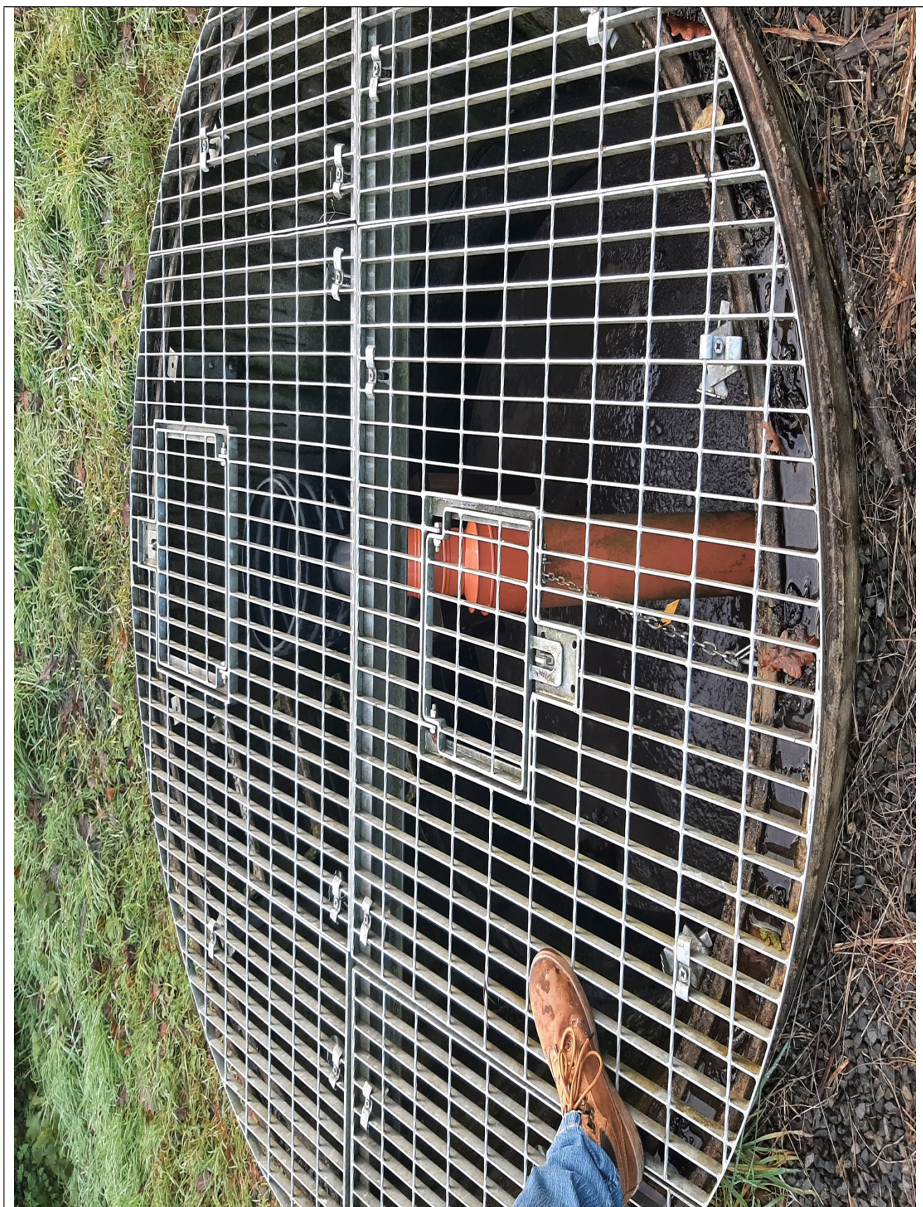
Above: Inspection chamber with cyclone system visible
