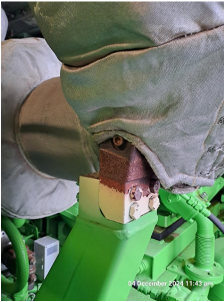
Current Stack Monitoring Location
