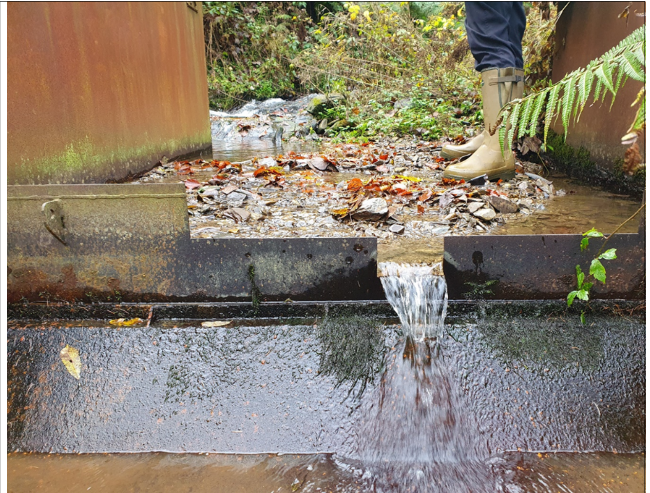
After - Full hands off flow notch level being achieved, with additional flow split through the compensation notch.
