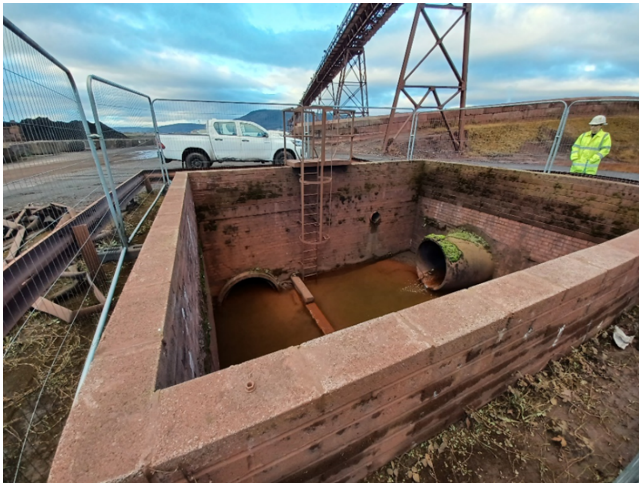
Image 6: W4 Sump - Monitoring Chamber
