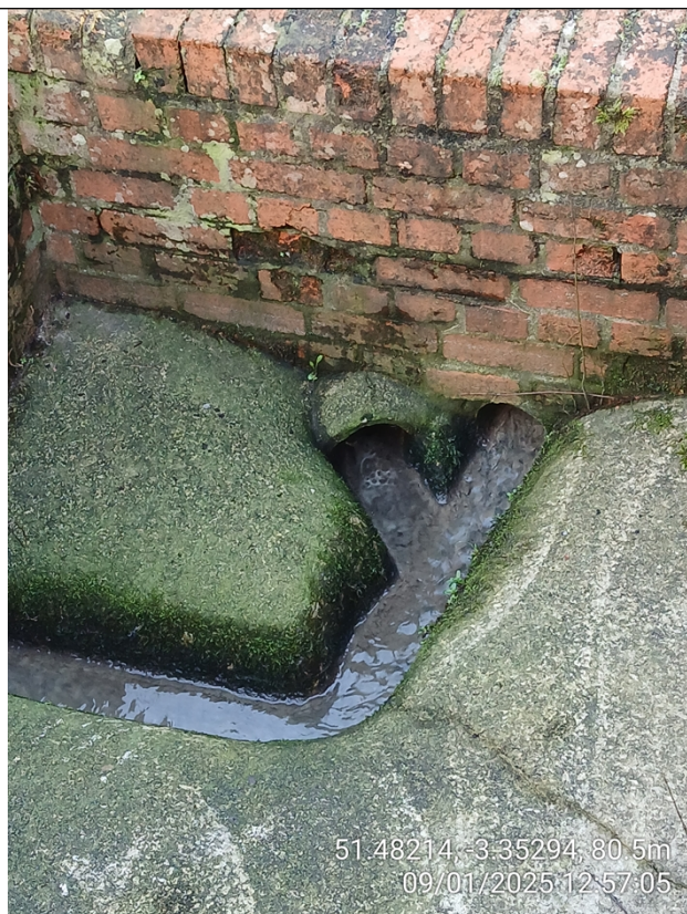
Humus tank (top), inlet pipe to humus (bottom).
