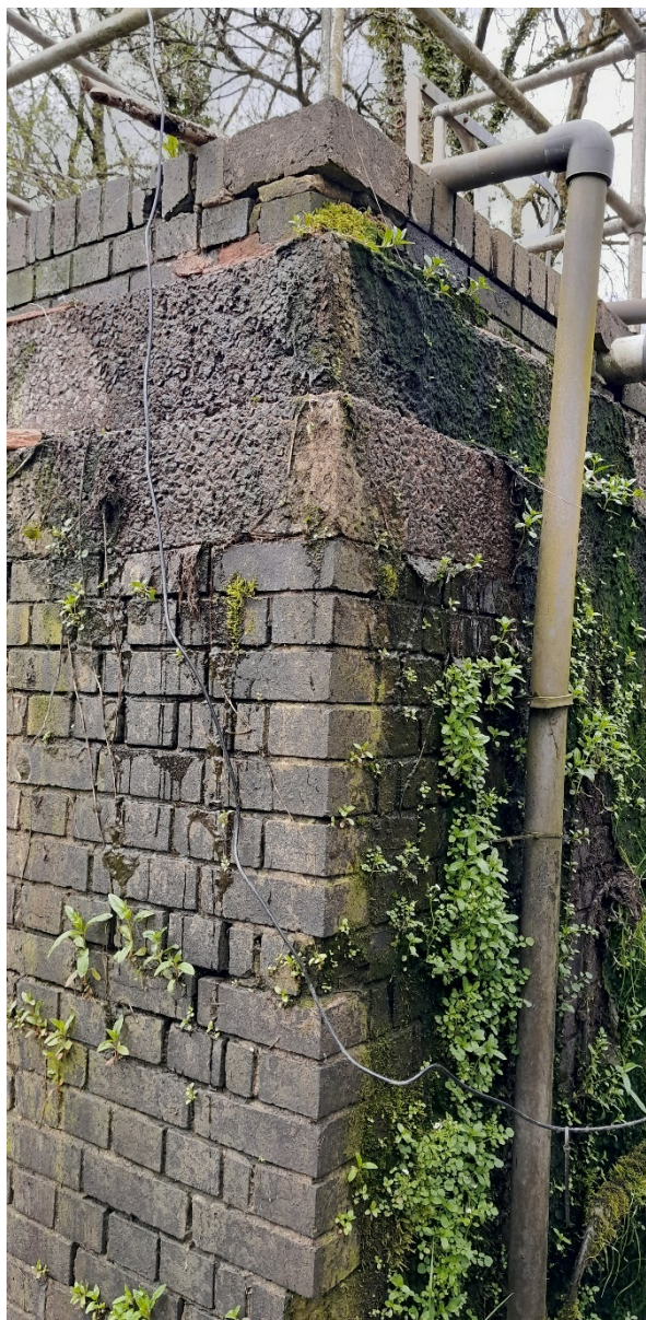
Figure 1: Distribution tank wall showing evidence of leaks.
