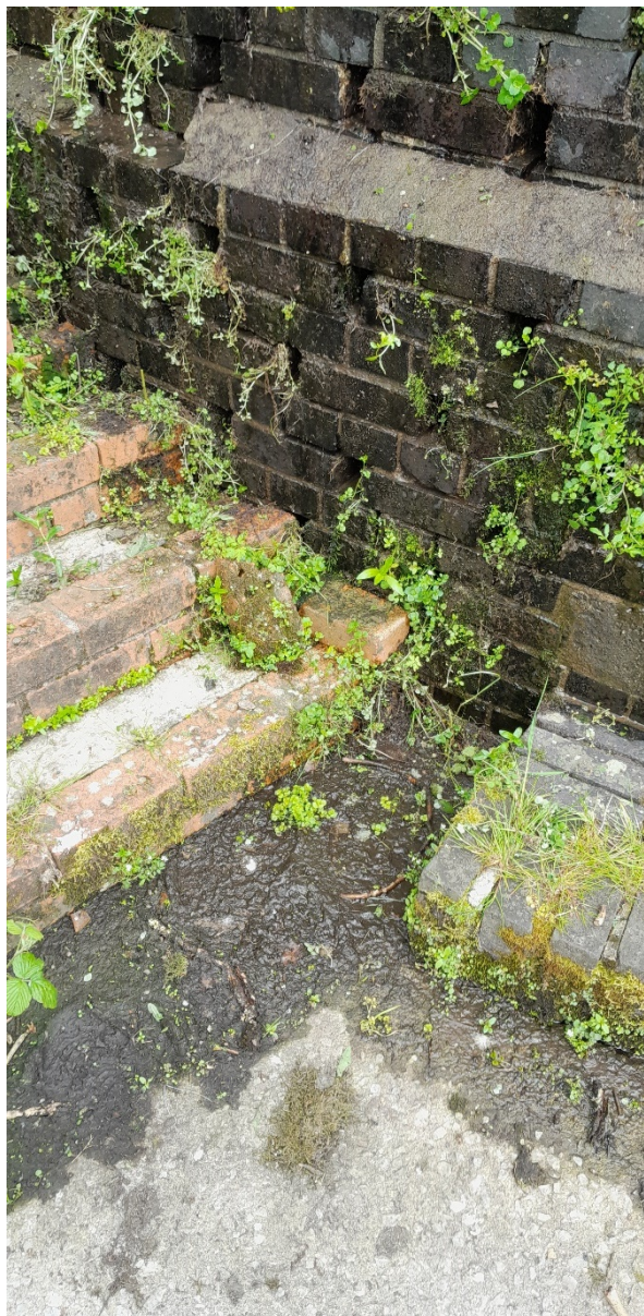
Figure 2: Leak from filter bed near steps.
