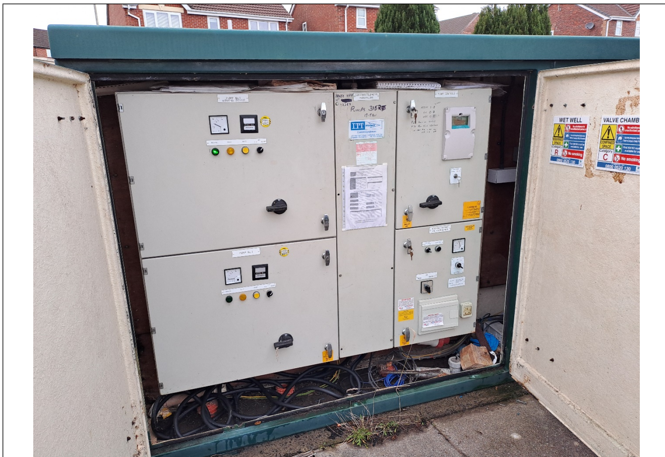
Figure 3 – System control box and telemetry
