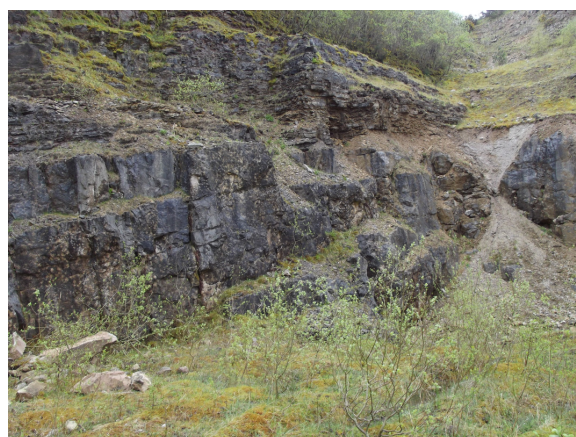
Plate 11: Ravelling failure at face corner
