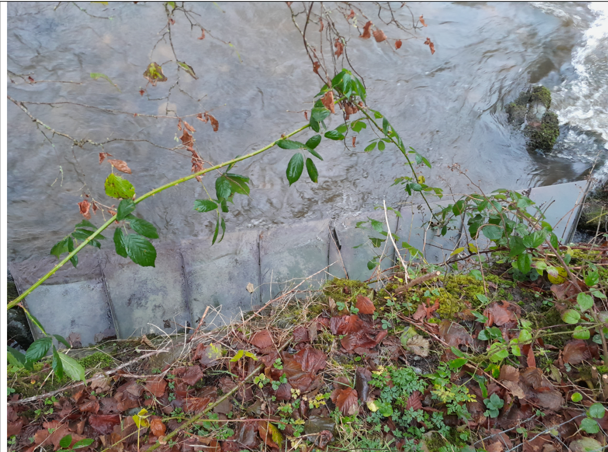
Photo 3. Discharge point below the turbine house - no apparent discharge.
