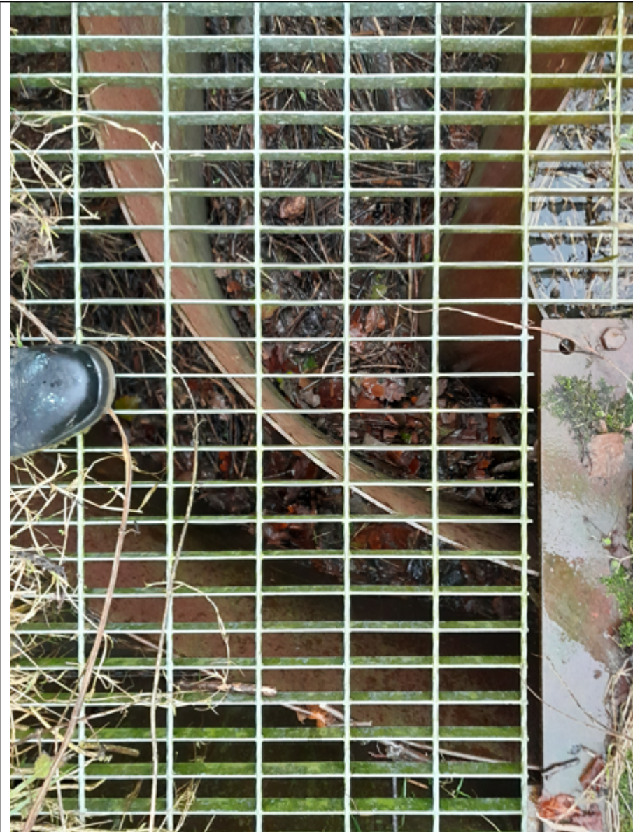
Photo 4. River debris accumulated in the bypass channels.
