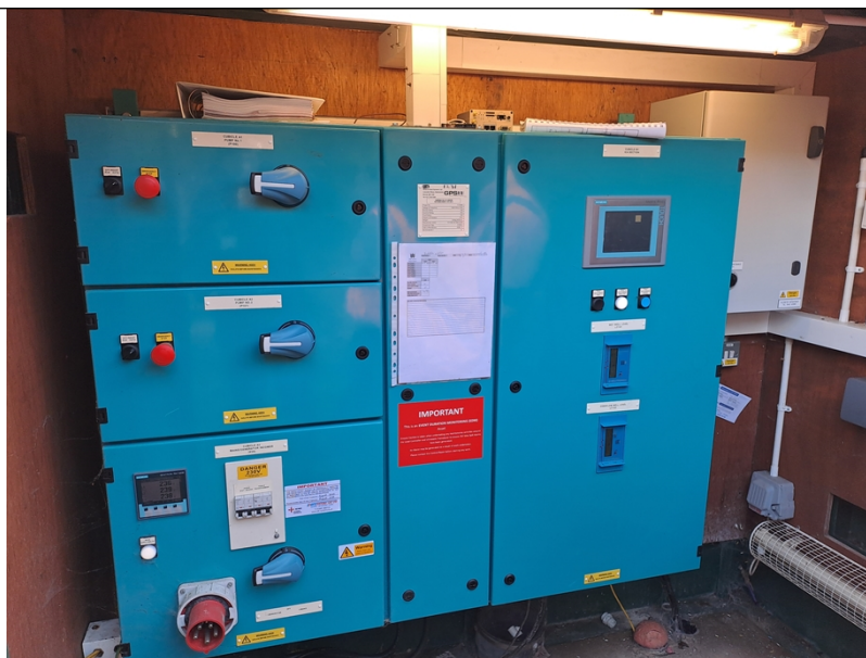
Figure 1: Site visit photo – Control box of the asset. Observed to be in good working order.
