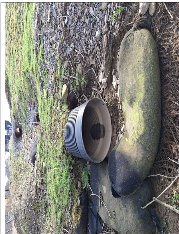
Figure 3: No discharge from discharge point 3
