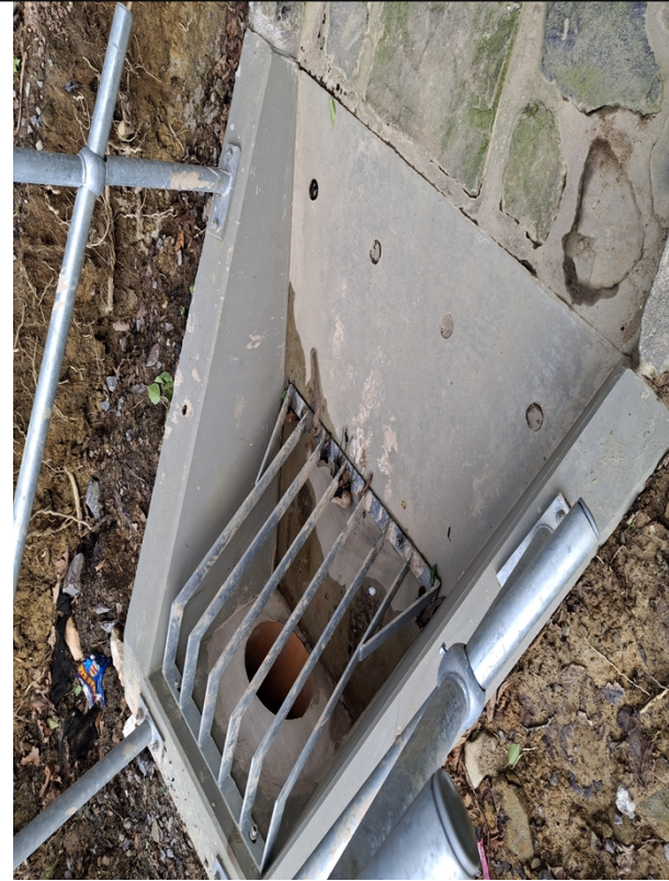
Figure 1: No discharge from discharge point 1
