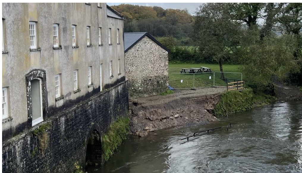
Figure 4. The wharf, photographed in 2023 after the collapse.
