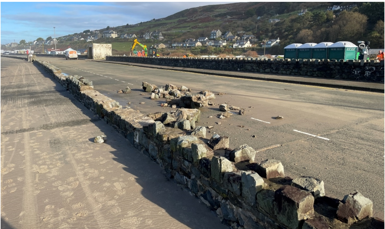
Photograph 10 View north showing storm damage to the stone wall dividing the promenade and roadway
