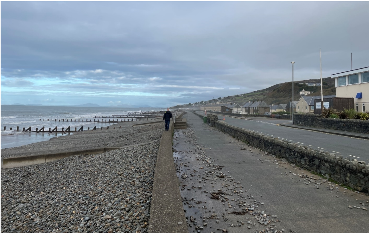
Photograph 1 View north along the promenade and roadway from the southern end of the site boundary. Shingle is covering the 1930s stone-faced apron wall.
