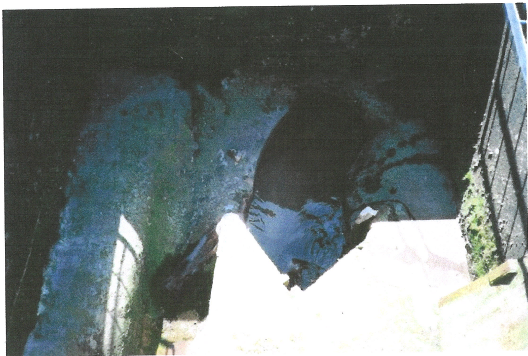
Photograph No.3 – View of chamber SH33802597, 300mm diameter inlet pipe to bifurcation chamber, overflow pipe to manually raked bar screen shown to the left.
