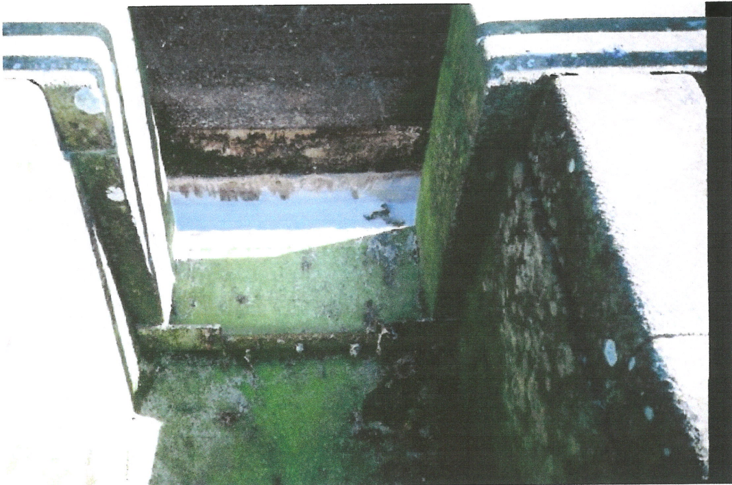
Photograph No.5 – Overflow weir from wet well
