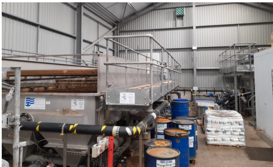
Image 1 – showing DAF within the enclosed building, taken on 3 October 2024
