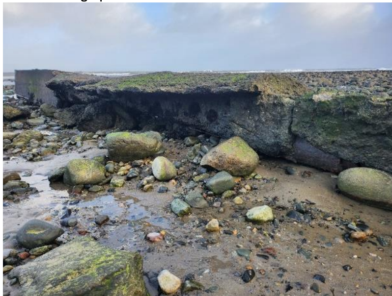
Site Photograph No 2 – Damaged pipe.
