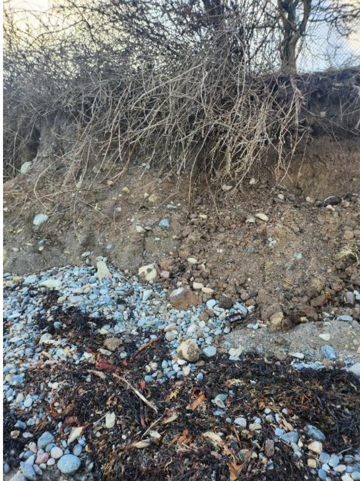
Site Photograph No 5 – Blackthorn on top of the cliff area.
