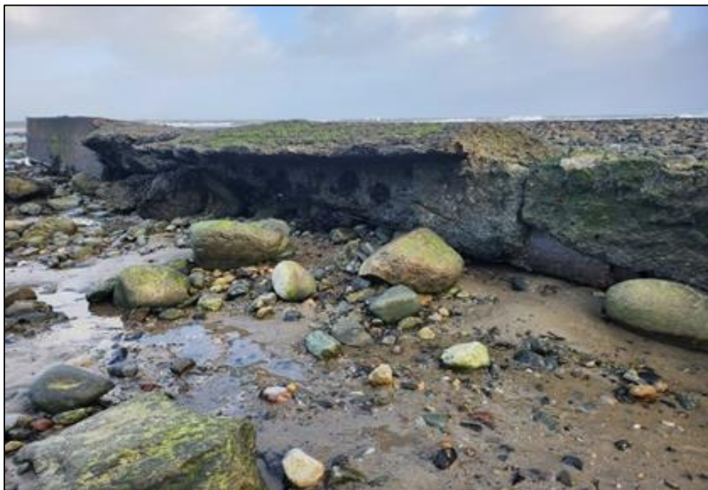
Figure 1: Damaged length of outfall pipe and concrete structure
