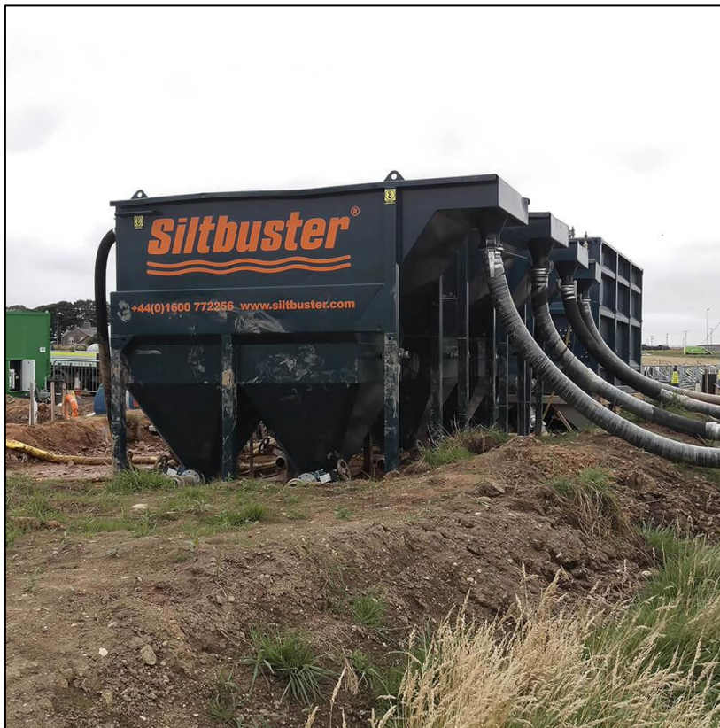
Figure 2 – Siltbuster Lamella Units in Parallel
