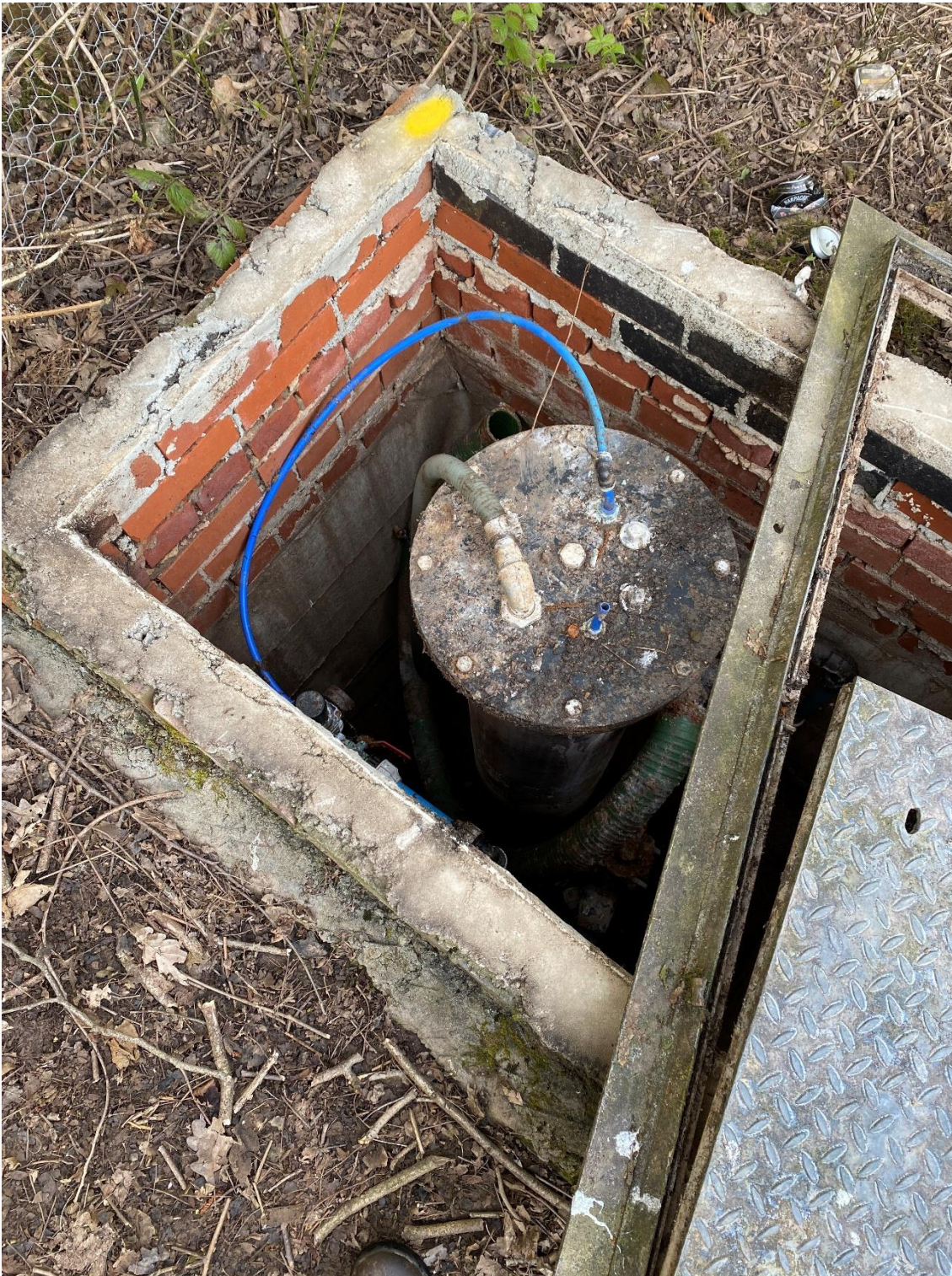
Figure 3.7: Leachate abstraction well LW10
