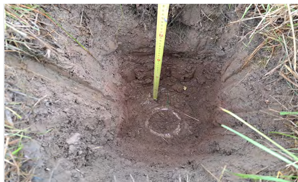
Plate 01: BH01 Redundant Clay Pipe at 0.60m bgl.
