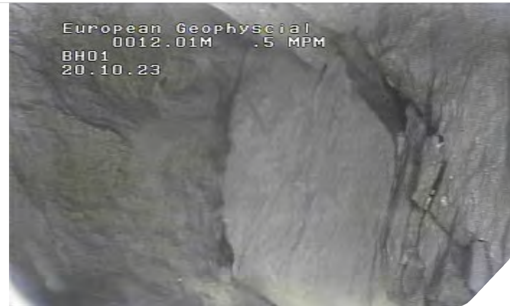
Plate 08: BH01 sidewall view at 12.01 m bgl. Irregular borehole sidewall, due to fracturing and collapse during drilling.
