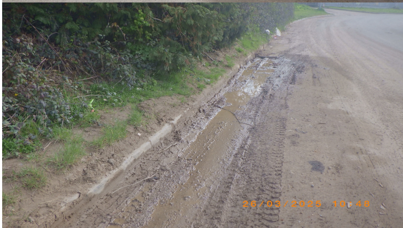
Photographs showing mud and debris leaving site & being tracked onto public highway
