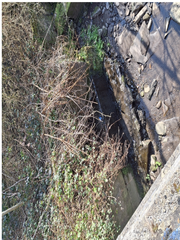
Figure 1: CSO discharging to the watercourse
