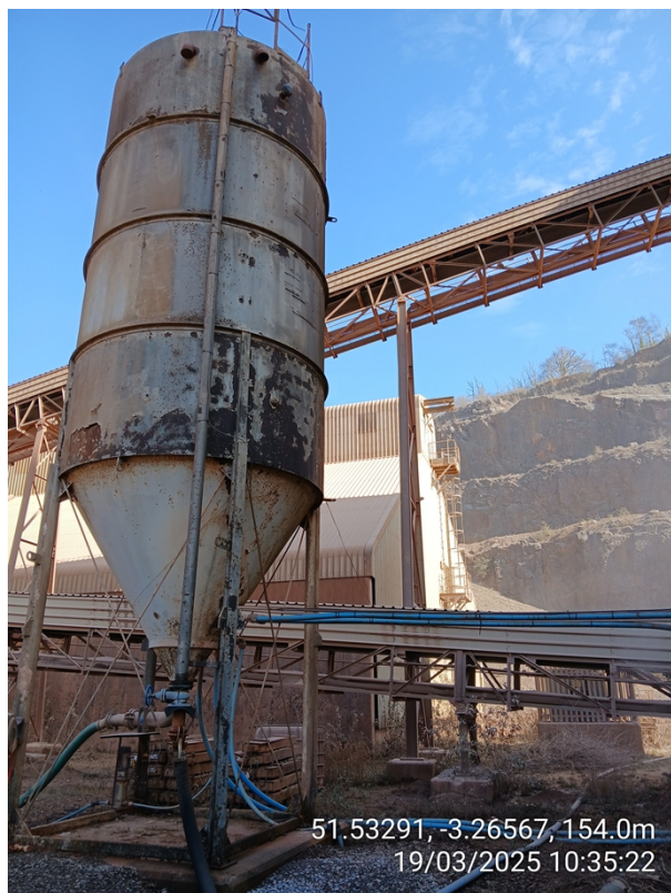
Water holding tank
