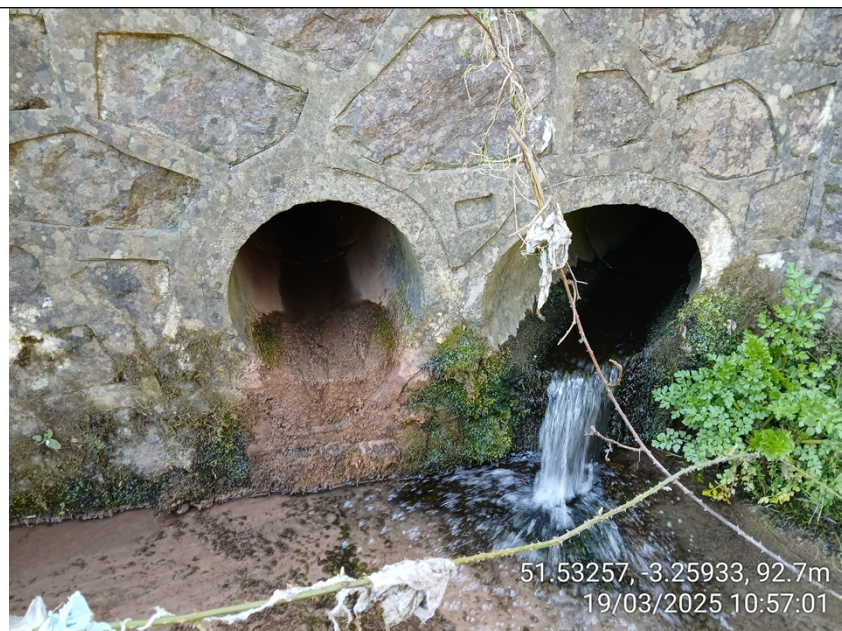
Outfall location: Left is quarry, Right is surface water.
