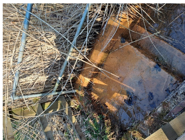
Figure 13 – Water overtopping the reedbed and flowing towards the discharge point due to vegetation build up.
