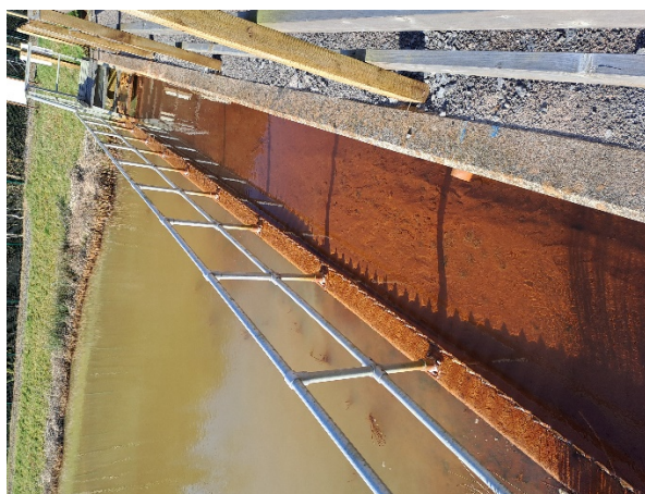
Figure 3 – Left hand outlet with significant sediment build up at the time of the visit.
