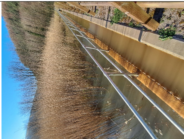
Figure 9 – The inlet to the reedbed as observed during the visit.
