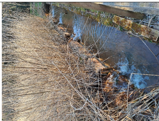
Figure 11 – Outlet of the reedbed showing build up of vegetation impacting flow.
