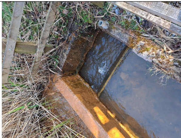
Figure 14 – The outlet from the reedbed at the time of the visit.
