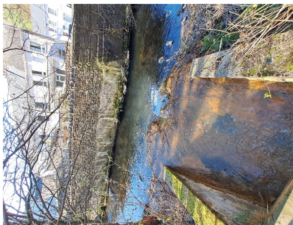
Figure 15 – The discharge point at the time of the visit.
