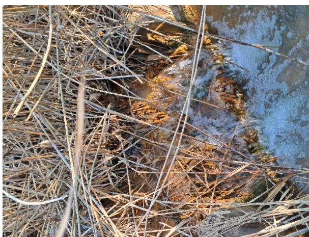
Figure 12 – One of the castellations with a build up of vegetation impacting flow.
