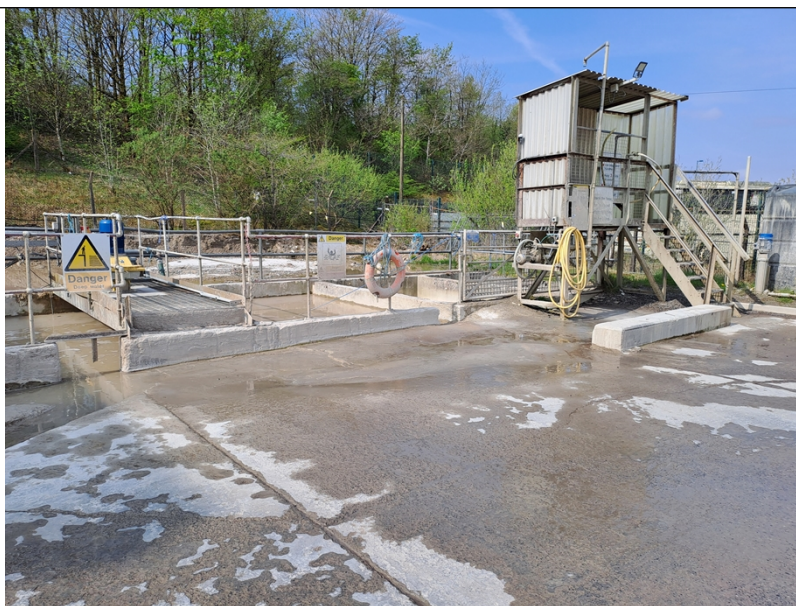
Figure 3 – Treatment tanks at the time of the visit with surface water drainage channels visible directing water into the treatment tanks.
