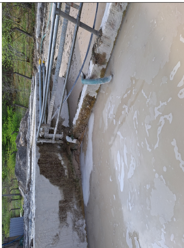
Figure 6 – A pipe used to channel excess surface water into the treatment tanks.
