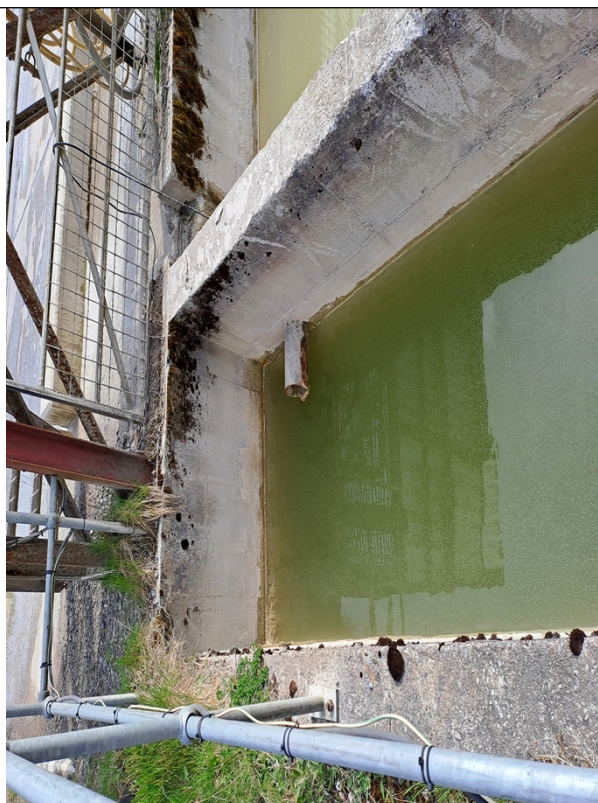
Figure 5 – The final settlement tank prior to discharge.
