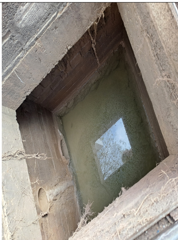
Figure 8 – Oil interceptor at the time of the visit.
