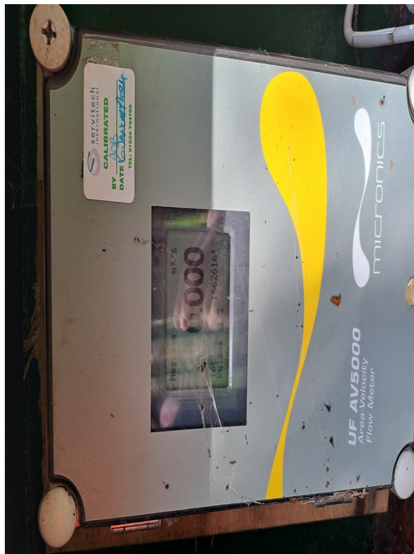
Figures 2 and 3 – Flow monitoring infrastructure at the time of the visit.
