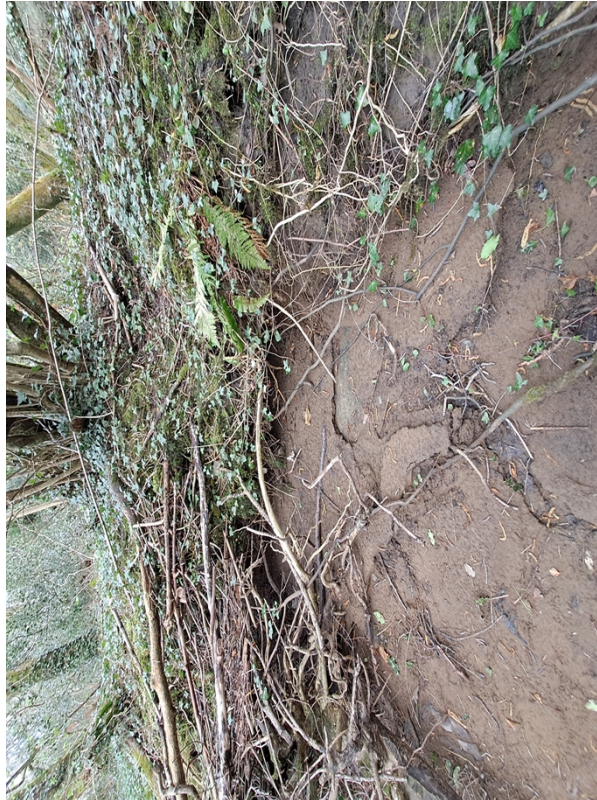
Figure 4 - The location of the outfall with evidence of flow seen in the sediments.
