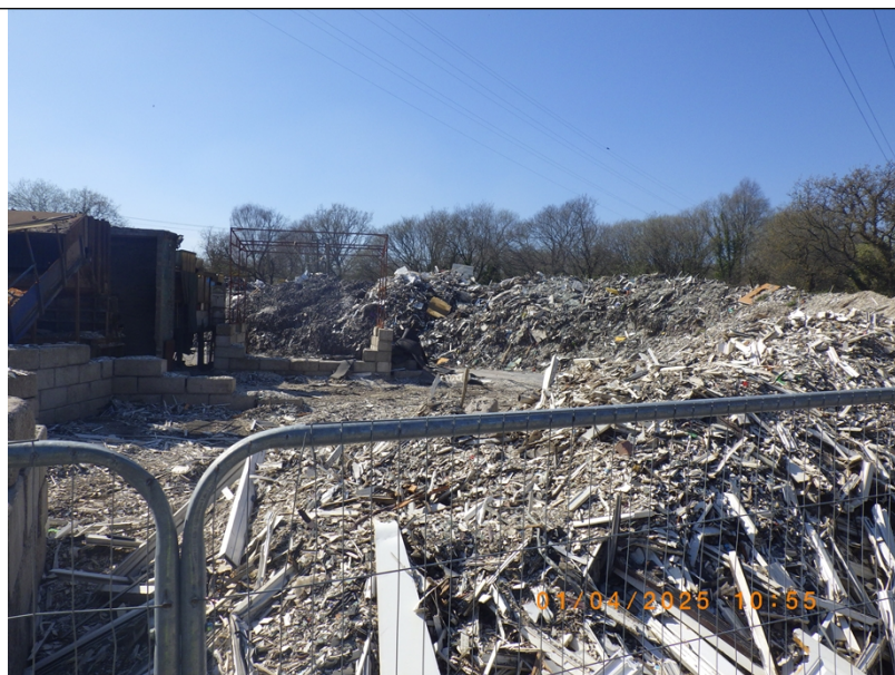
Image 2 - storage of waste at the front of the site with no fire breaks installed and not in line with the submitted FPMP.
