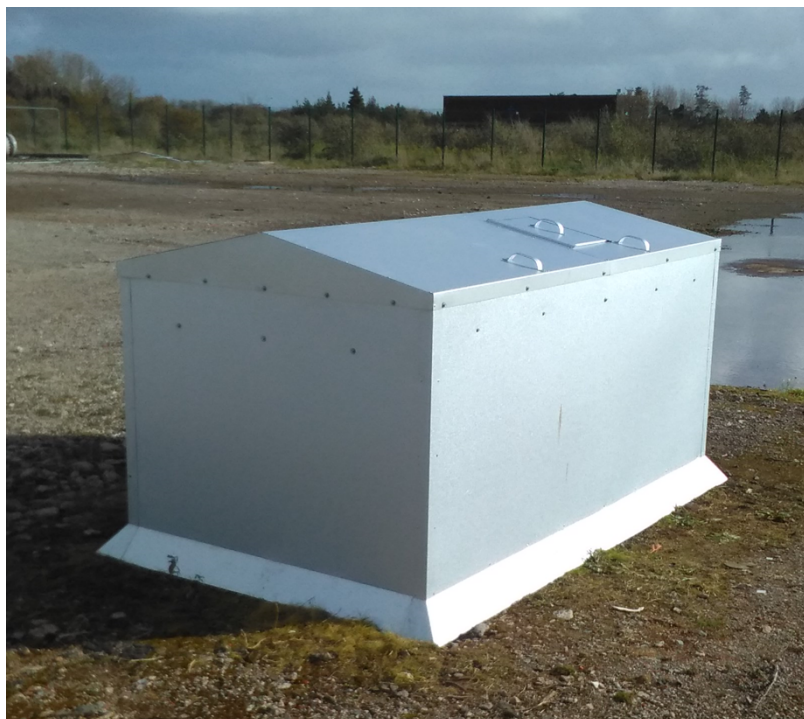
South Pit enclosure with accessible inspection and sampling point
