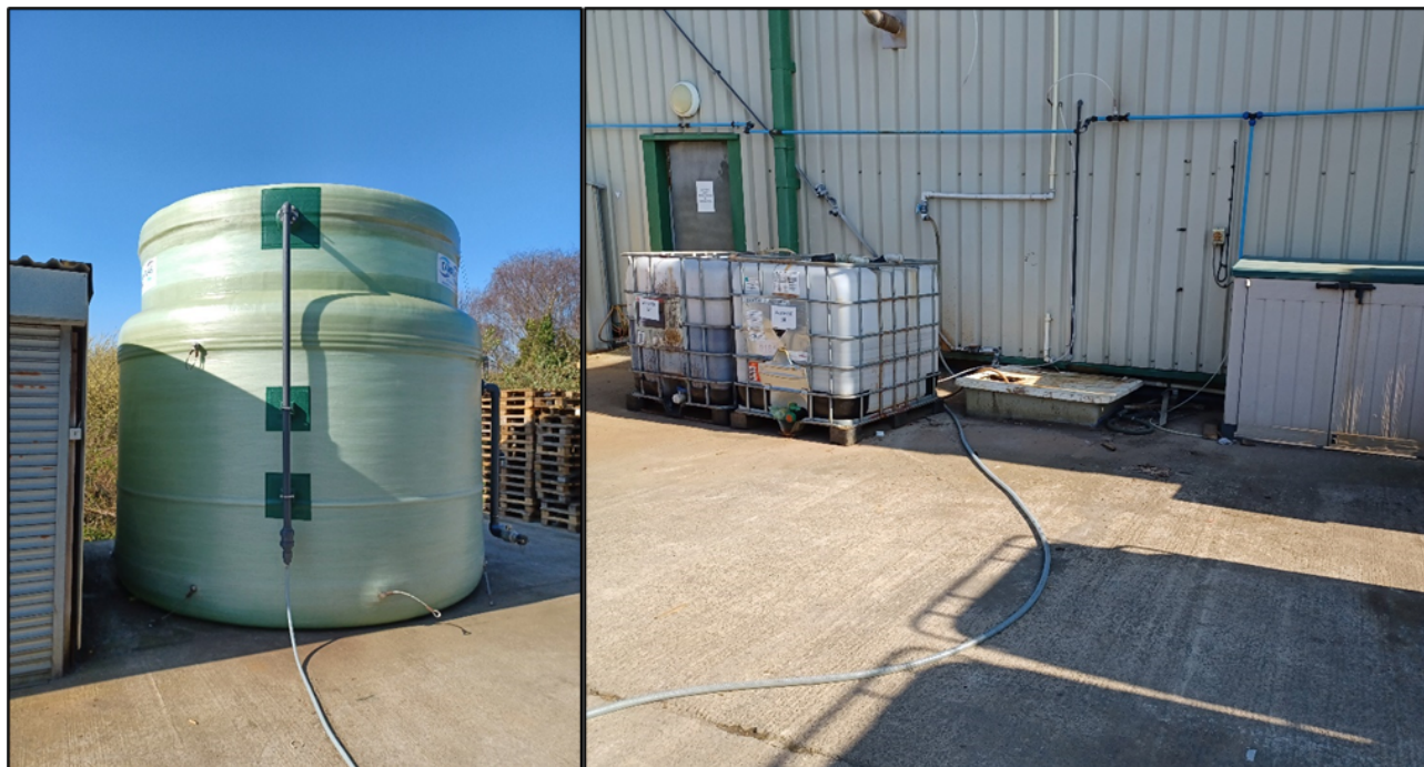
Images 1 and 2: Integrally banded wastewater tank and inlet pipework entering via reception sump (right).
