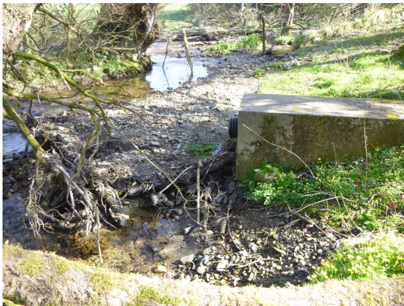
Photograph 2: Storm and emergency discharge point into Nant Collen at SN 34608 47317
