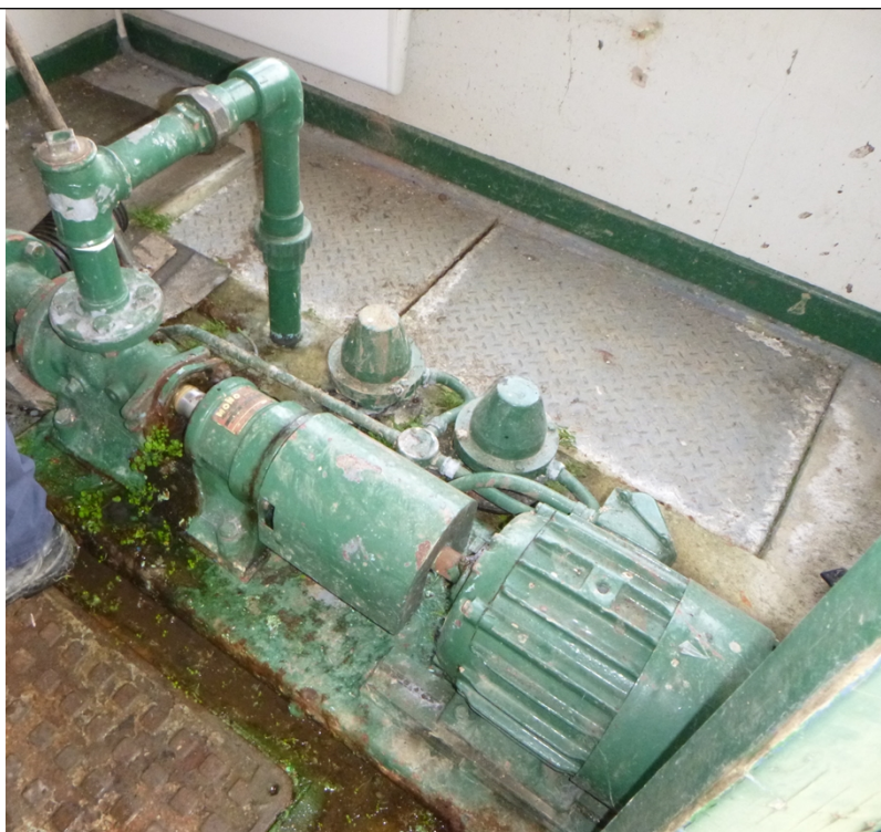
Photograph 8: Self-lubricating pump within the site's control room
