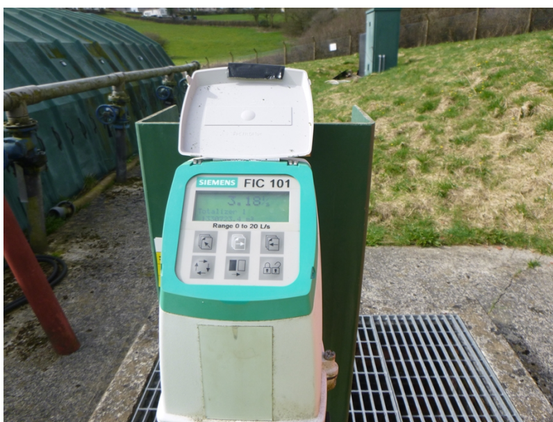
Photograph 3: Flow meter recording flows to full treatment
