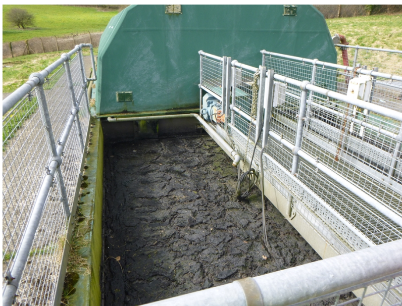
Photograph 5: Final settlement tank
