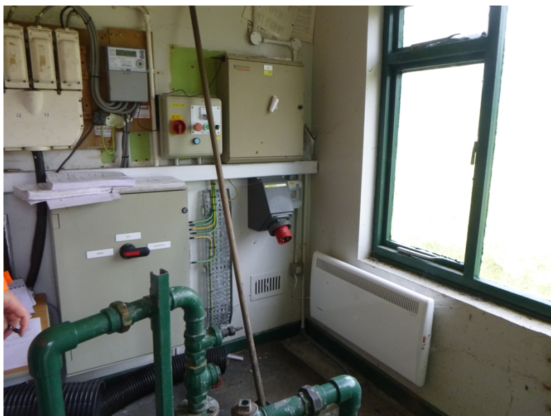
Photograph 9: Generator socket in Beulah WwTW's control room
