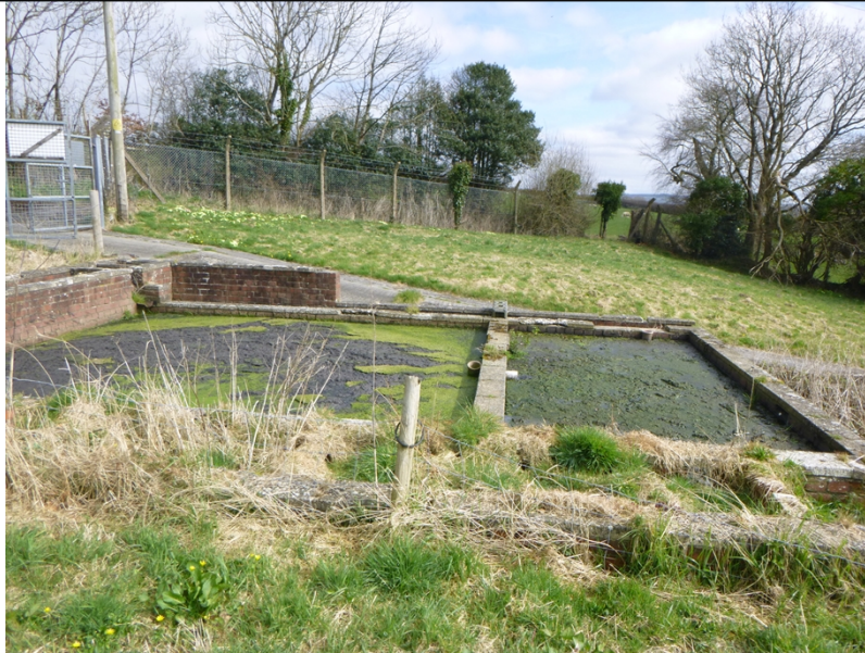
Photograph 6: Sludge holding tank at Beulah WwTW
