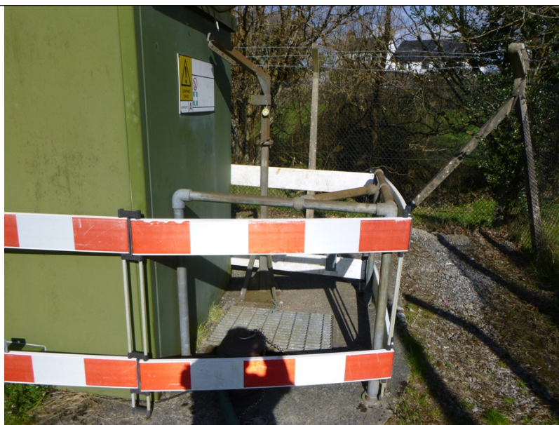
Photograph 2: Pumping station at Rhydlewis WwTW. Wet well exists below grate.
