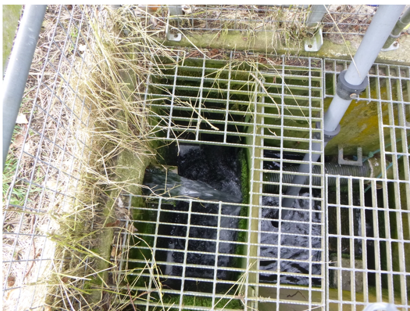
Photograph 9: Final effluent sample point and turbidity probe
