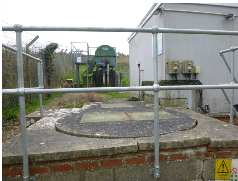
Photograph 1: Inlet chamber with screen visible in background
