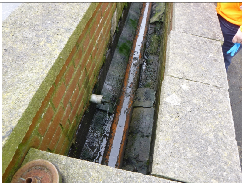
Photograph 8: Effluent discharge from sludge holding tanks
