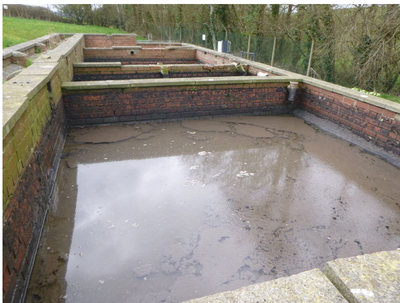
Photograph 7: Sludge holding tanks
