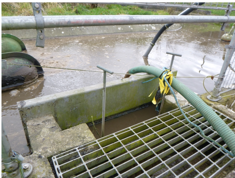
Photograph 5: Activated sludge return pipe
