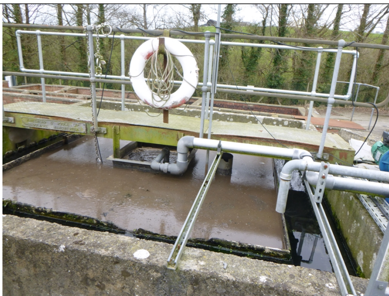
Photograph 4: First settlement tank
