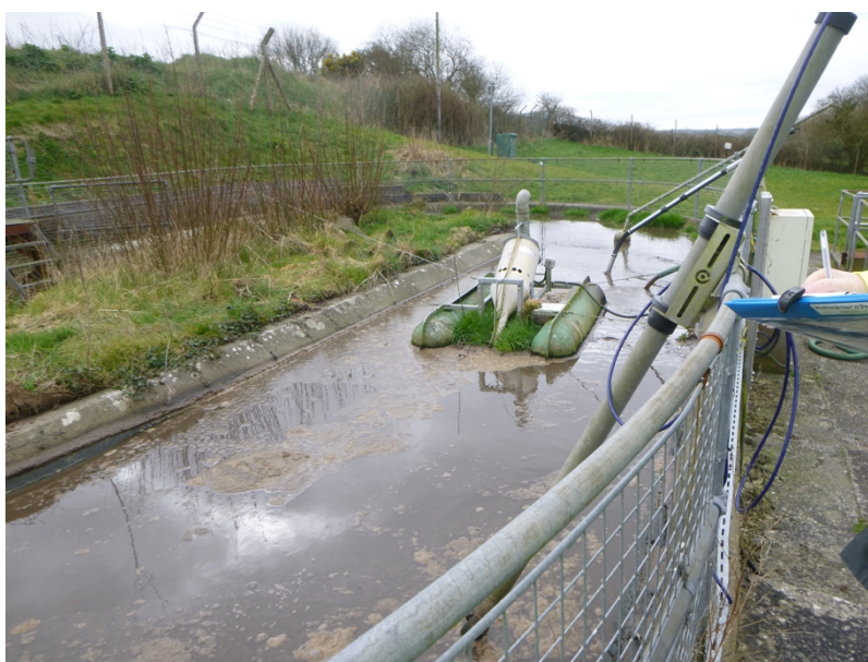
Photograph 3: Aeration lane with mobile aerator
