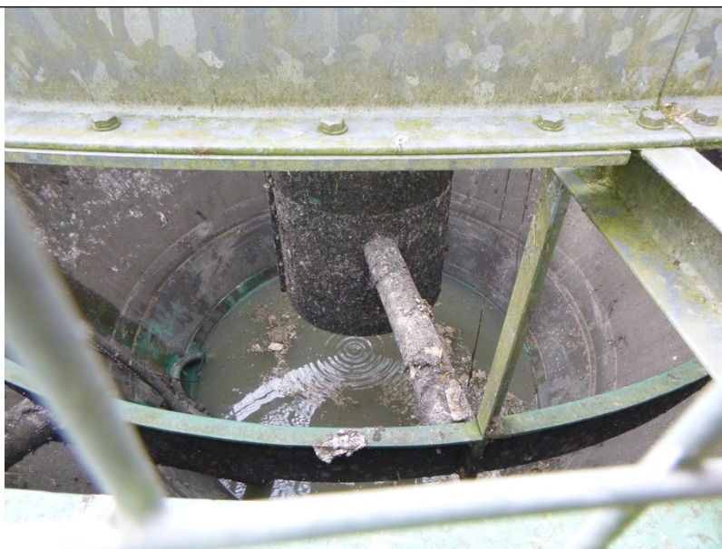
Photograph 2: Conical storm tank
