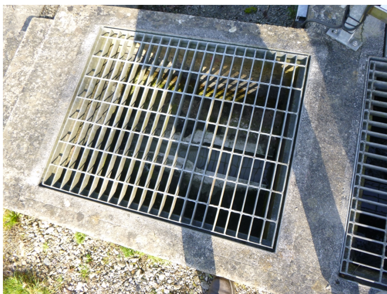
Photograph 1: Rhydlewish WwTW inlet
