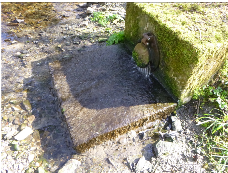
Photograph 5: Final effluent outfall into the Nant Collen. Sewage fungus present on outfall wall.
