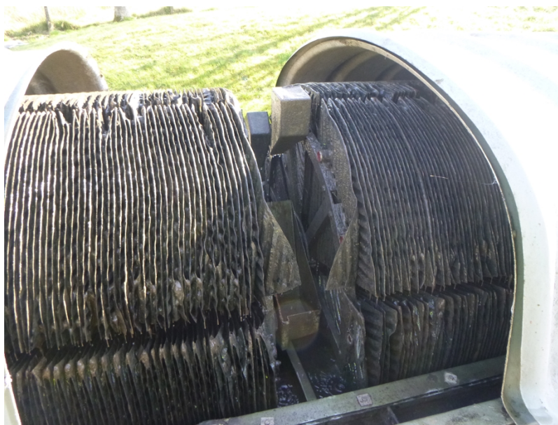
Photograph 2: Discs of Rotating Biological Contractor (RBC)
