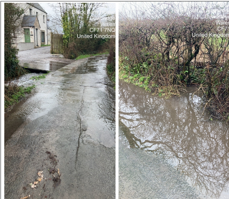
Left: Stembridge brook breaking its banks; Right: blocked culvert found at NGR SS 96576 73715
